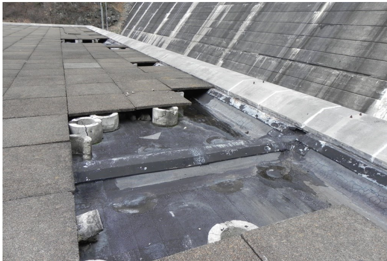
Perimeter coping, roof pavers, pedestals, and nailable concrete cants over construction joints. The roof membrane is visible where pavers are displaced.
