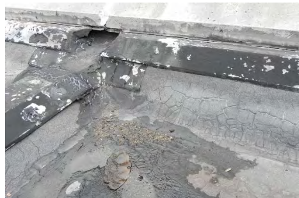
Base flashing and sheet metal flashing at construction joint and perimeter coping
