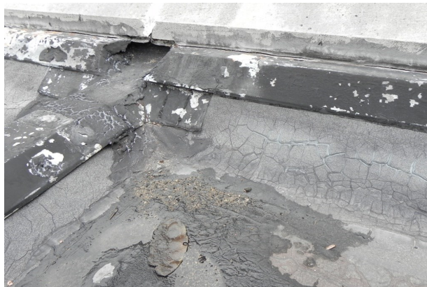
Base flashing and sheet metal flashing at construction joint and perimeter coping
