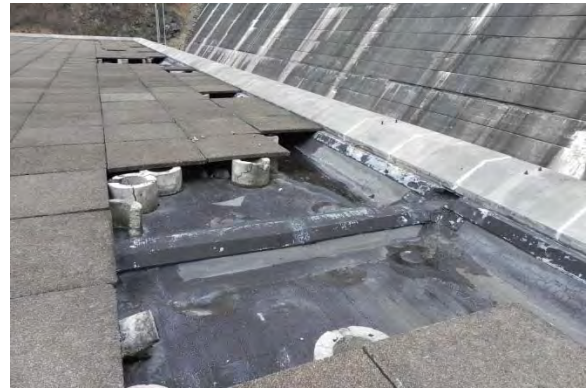
Perimeter coping, roof pavers, pedestals, and nailable concrete cants over construction joints. The roof membrane is visible where pavers are displaced.
